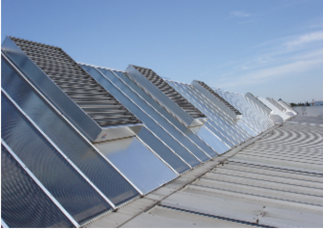
SMOKEJET in shed roof glazing
