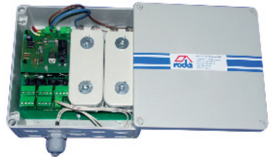
SHE-Box with nickel-cadmium batteries granting an emergency power supply in case of SHE-triggering due to heat or smoke.
