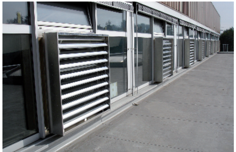
SMOKEJET in vertical glazing
