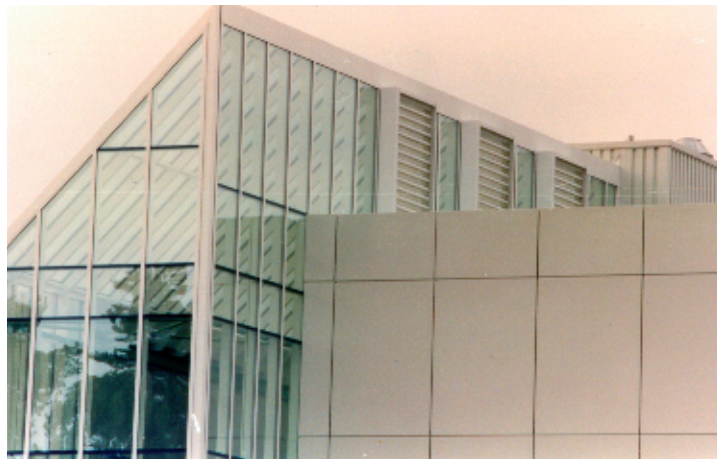
SMOKEJET in vertical glazing
