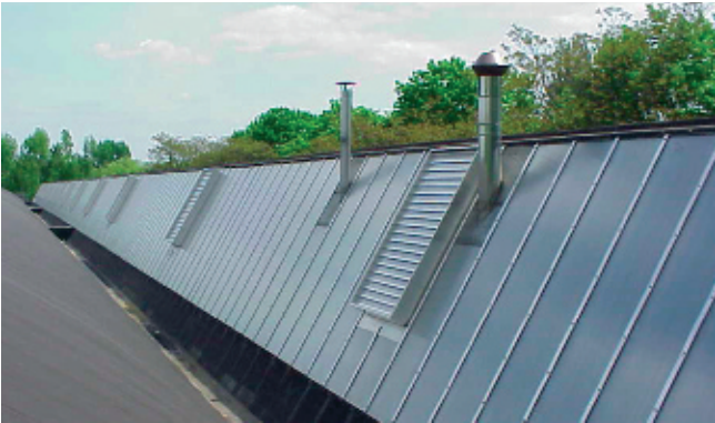
SMOKEJET in shed roof glazing
